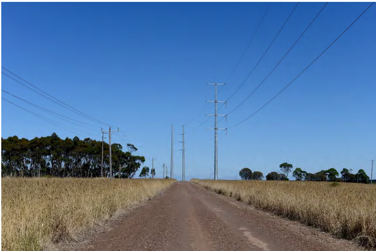
Plate 7 – View toward existing transmission line infrastructure including angle poles, Mortlake (Image: ©GBD 2023)
