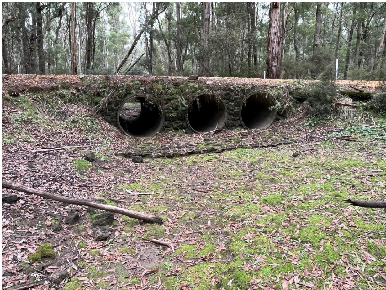
Figure 7 Dry riverbed in Surrey River at Boiler Swamp Road (central crossing site) on 20 April 2023
